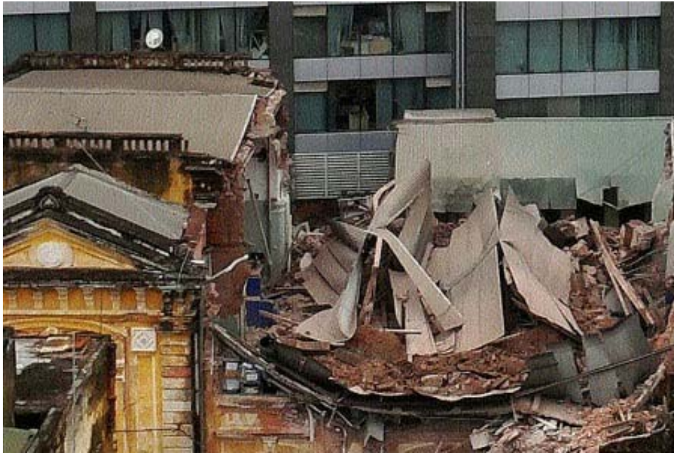
Sudden: The recent house collapse on Tran Hung Dao Street.
